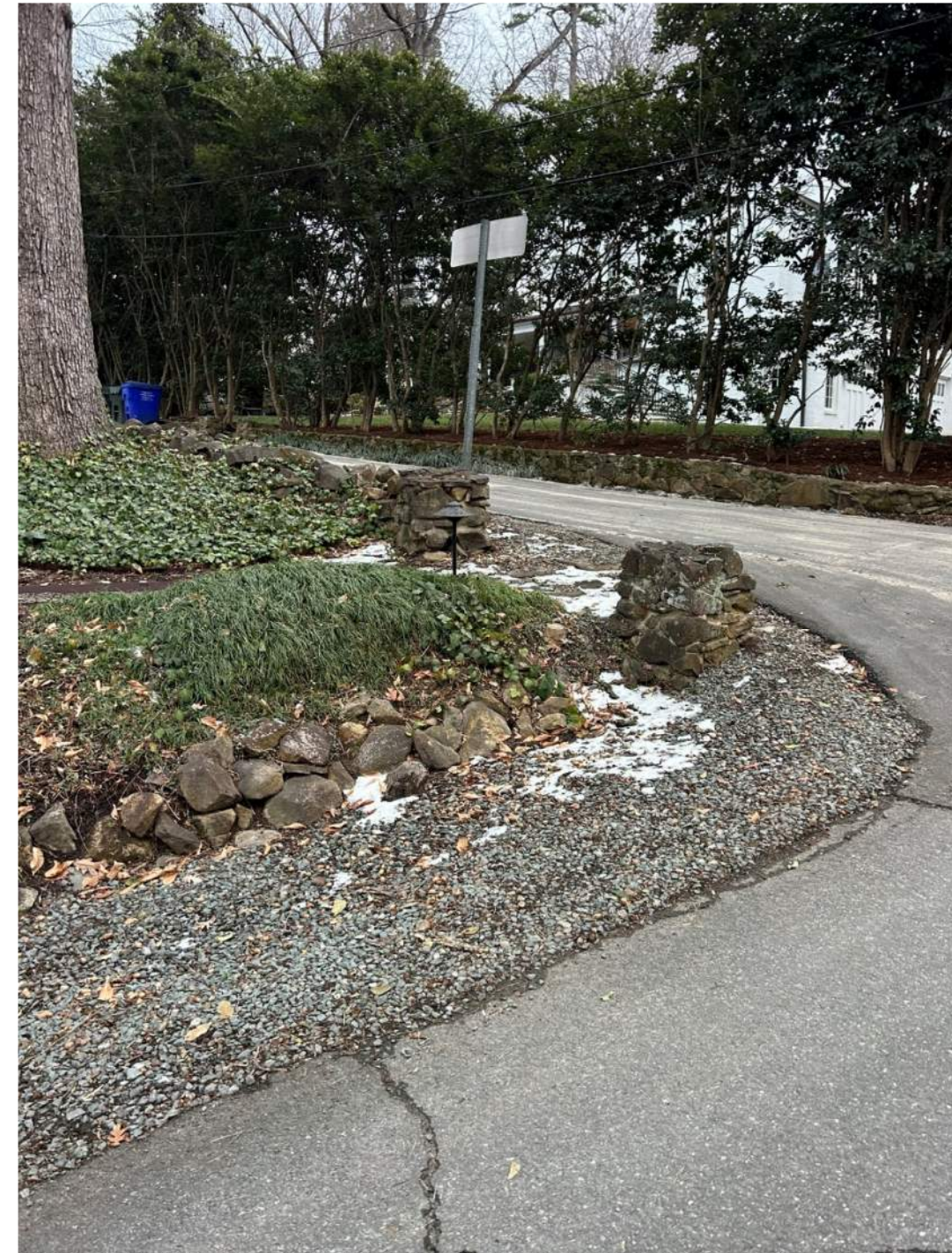
Existing Stone Columns @ corner of Glandon/Evergreen (repair)
