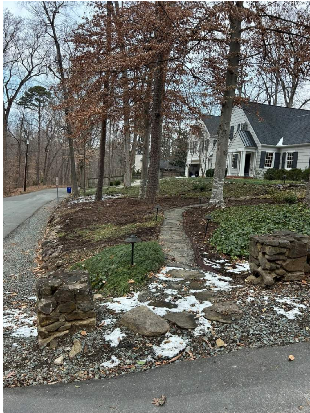
Existing Stone Columns @ corner of Glandon/Evergreen (repair)
