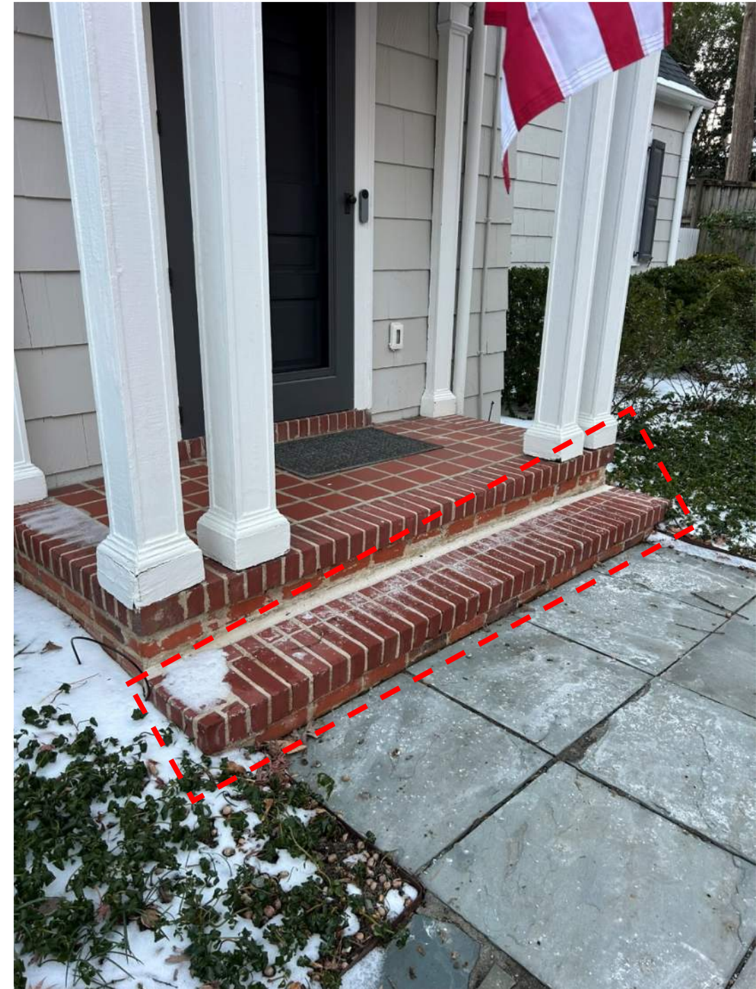
Existing Front Stoop step (to be replaced in-kind)
