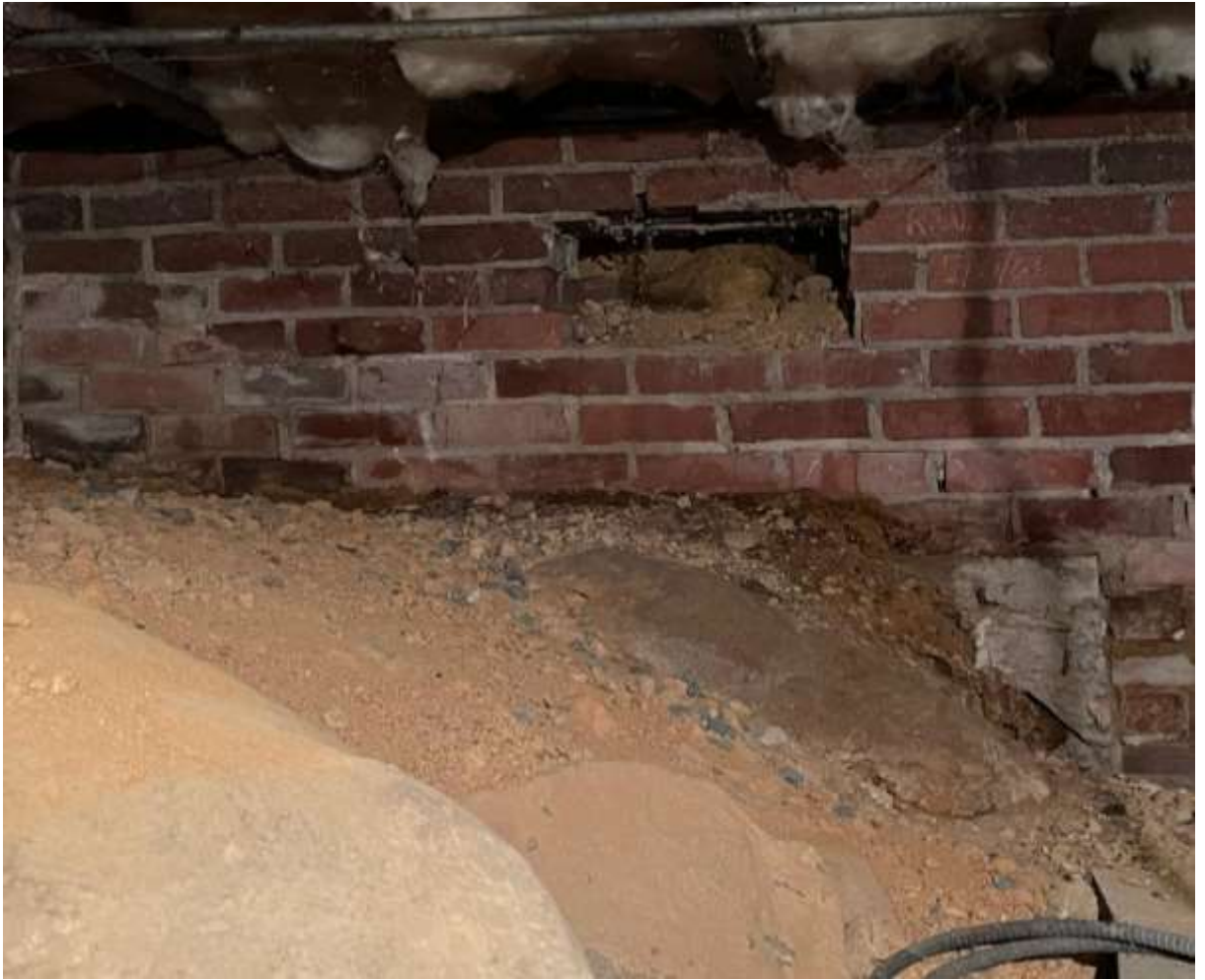
Figure 43 – Internal View of Basement - Vents
