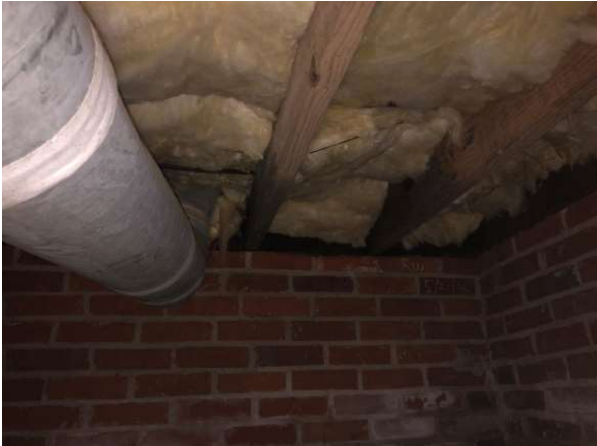
Figure 47 - Evidence of wood floor joist in contact of brick wall suffering deterioration (black and humid appearance)
