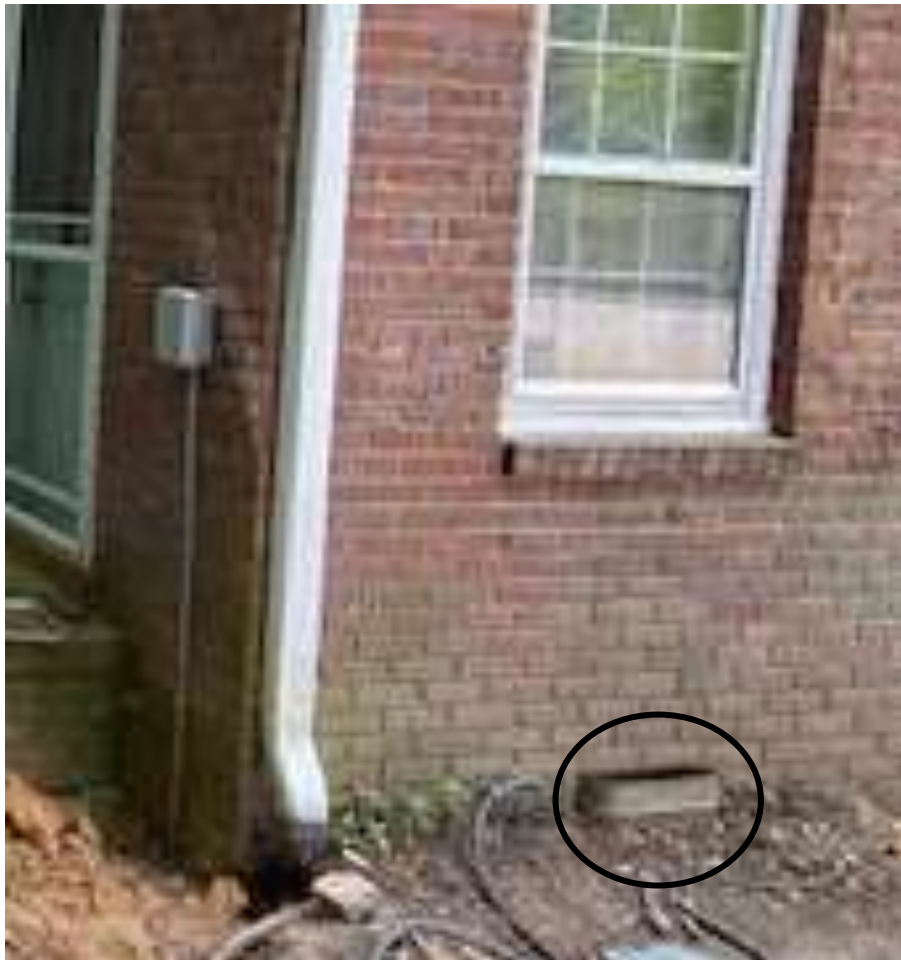
Figure 42 – Basement Vents (Black Circle)
