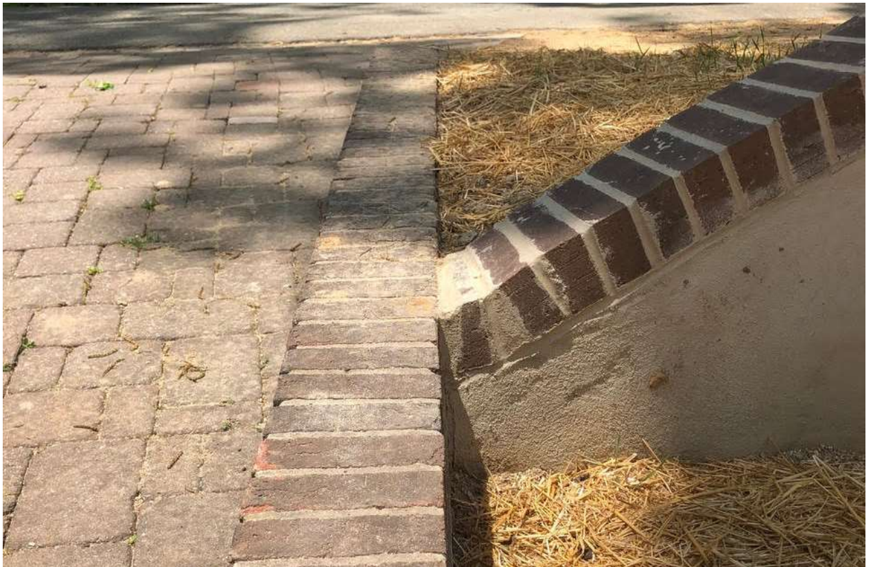
Figure 60 - New Brick Cap of Retaining Wall Meeting Existing Brick Wall on the Edge of the Driveway
