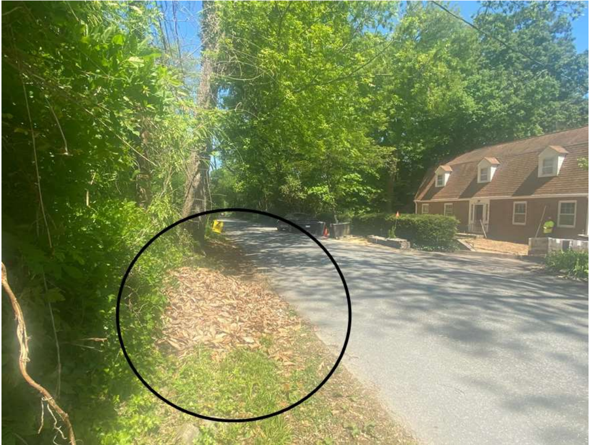
Figure 38 – Evidence of green material and occasional debris on the side of Hooper Lane
