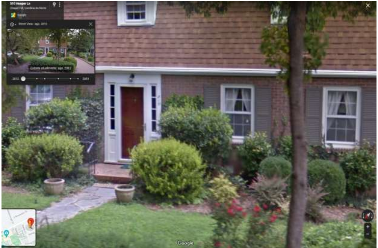
Figure 33 - Vegetation on masonry
