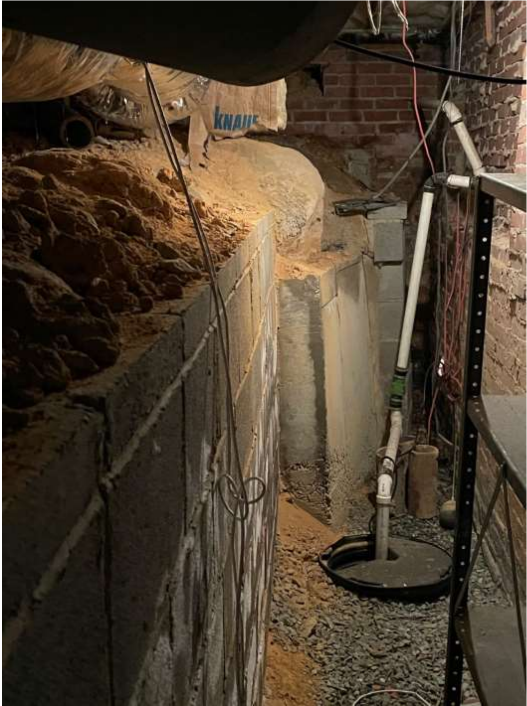
Figure 45 – Northeast side view of the basement (Evidence of a Block wall and a Poured Concrete Wall).
