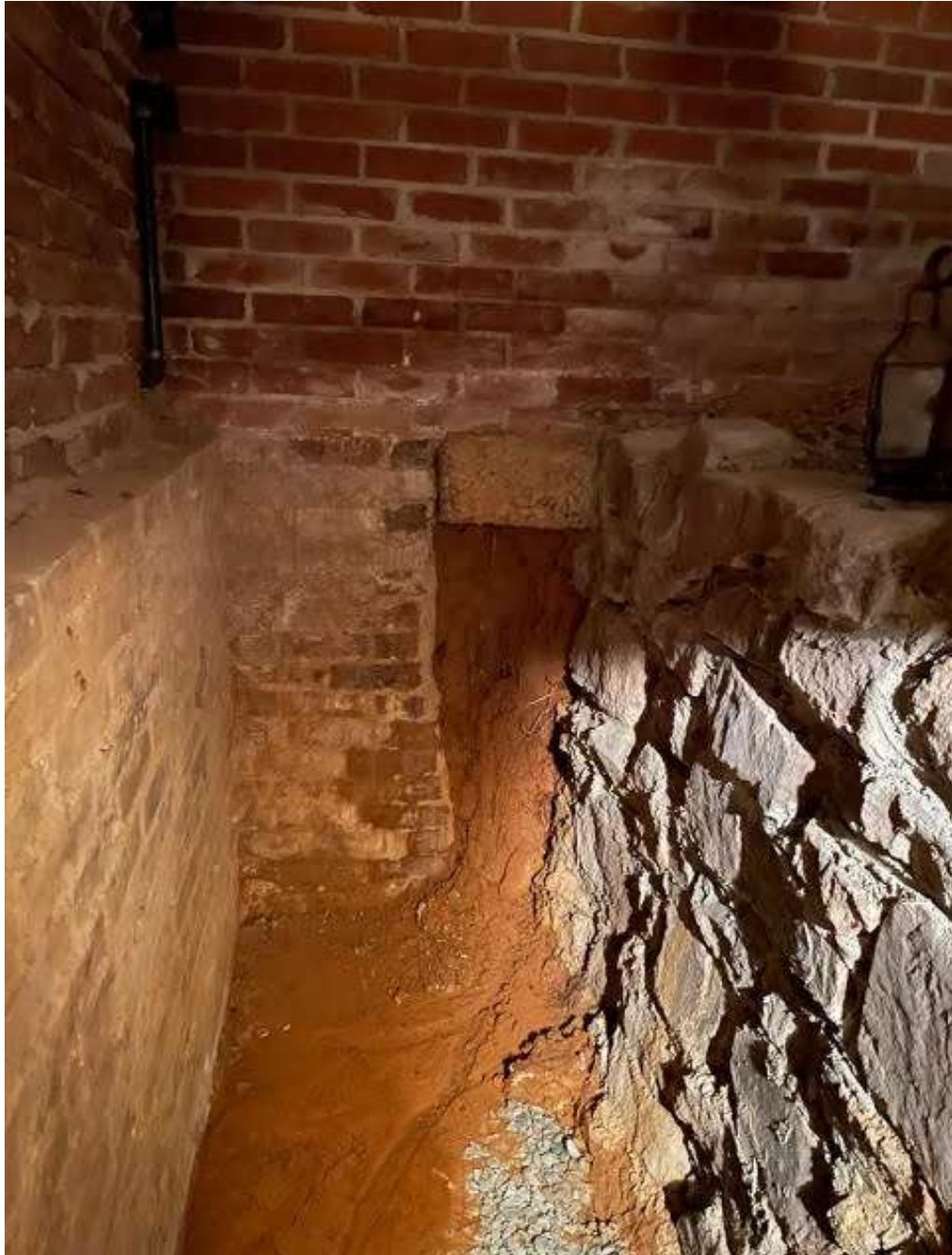
Figure 44 – Northwest side view of the basement (soil sliding).
