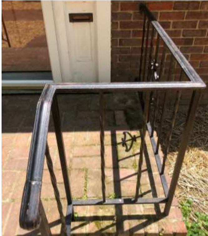
Figure 73 - Existing Metal Railing to be Used as Reference for new railing to be installed on front steps.
