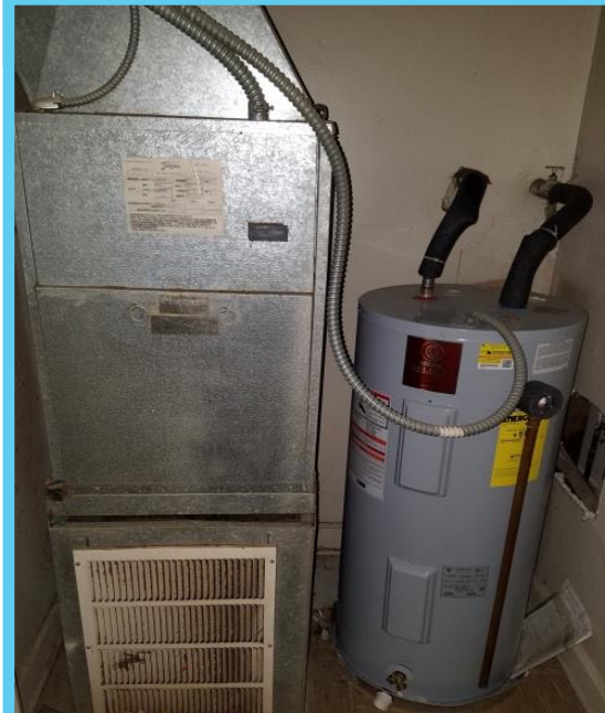
Typical existing furnace
