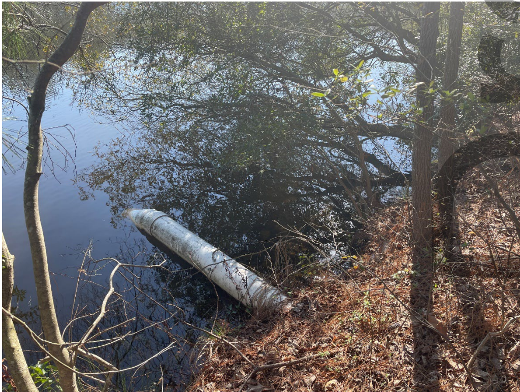
Photograph 4 – PVC Overflow Device Inlet
