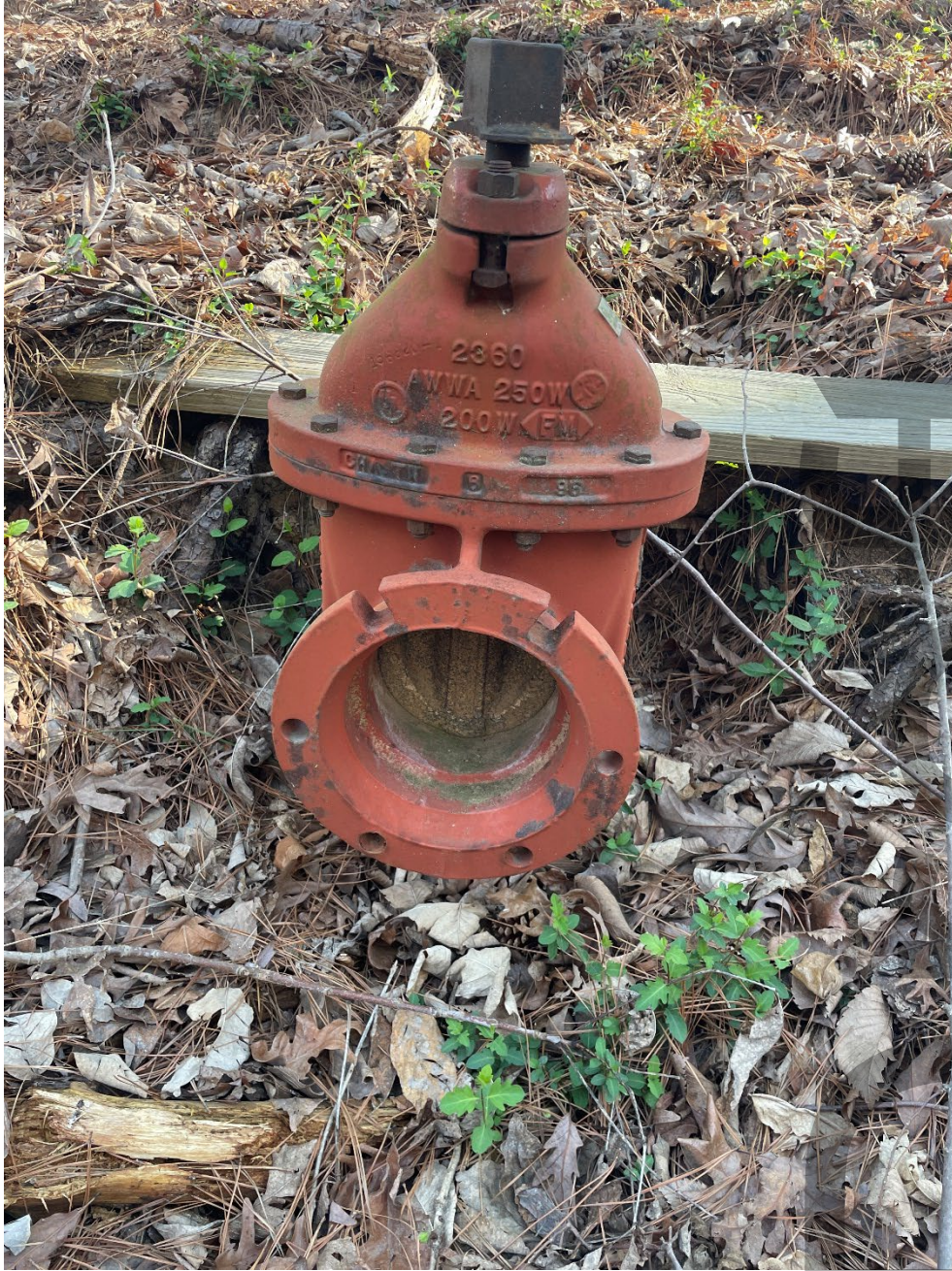
Photograph 7 – Butterfly Valve at Downstream End of Primary Outlet
