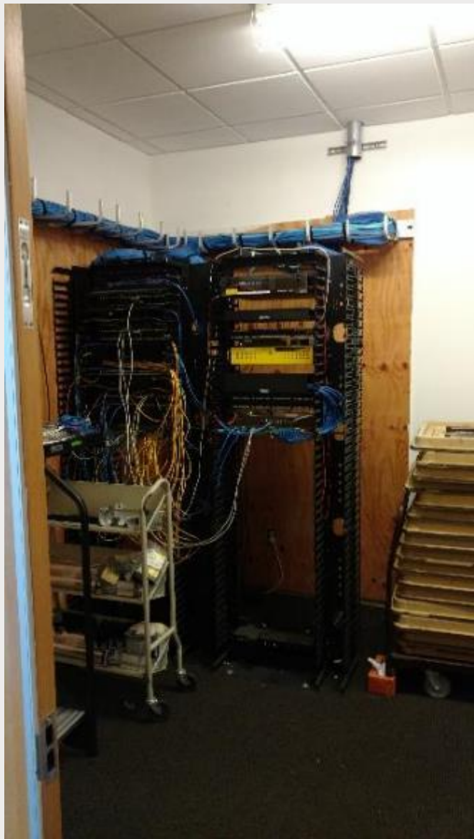
Equipment racks in facilities
