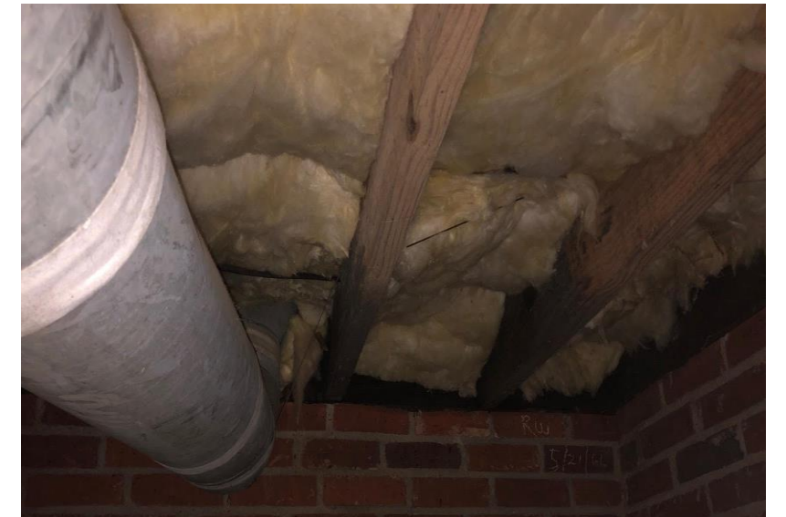
Image 4 | Timber Structure (Dark Colored Section in Contact with Brick Wall)
