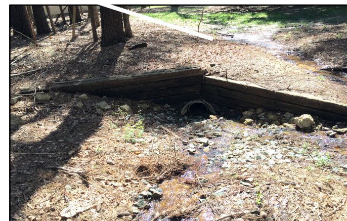
12" Stormwater Pipe Inlet Summerfield Crossing Property
