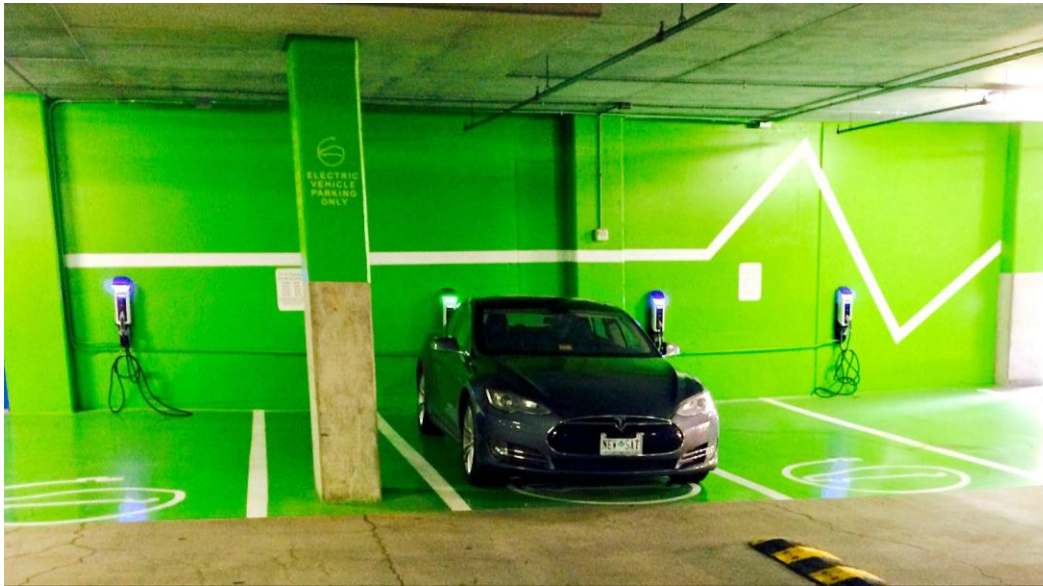
EV charging stations
