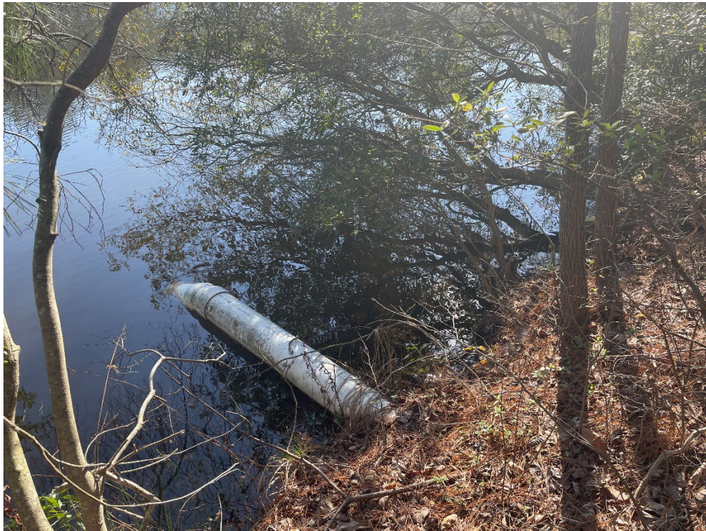
Photograph 4 – PVC Overflow Device Inlet
