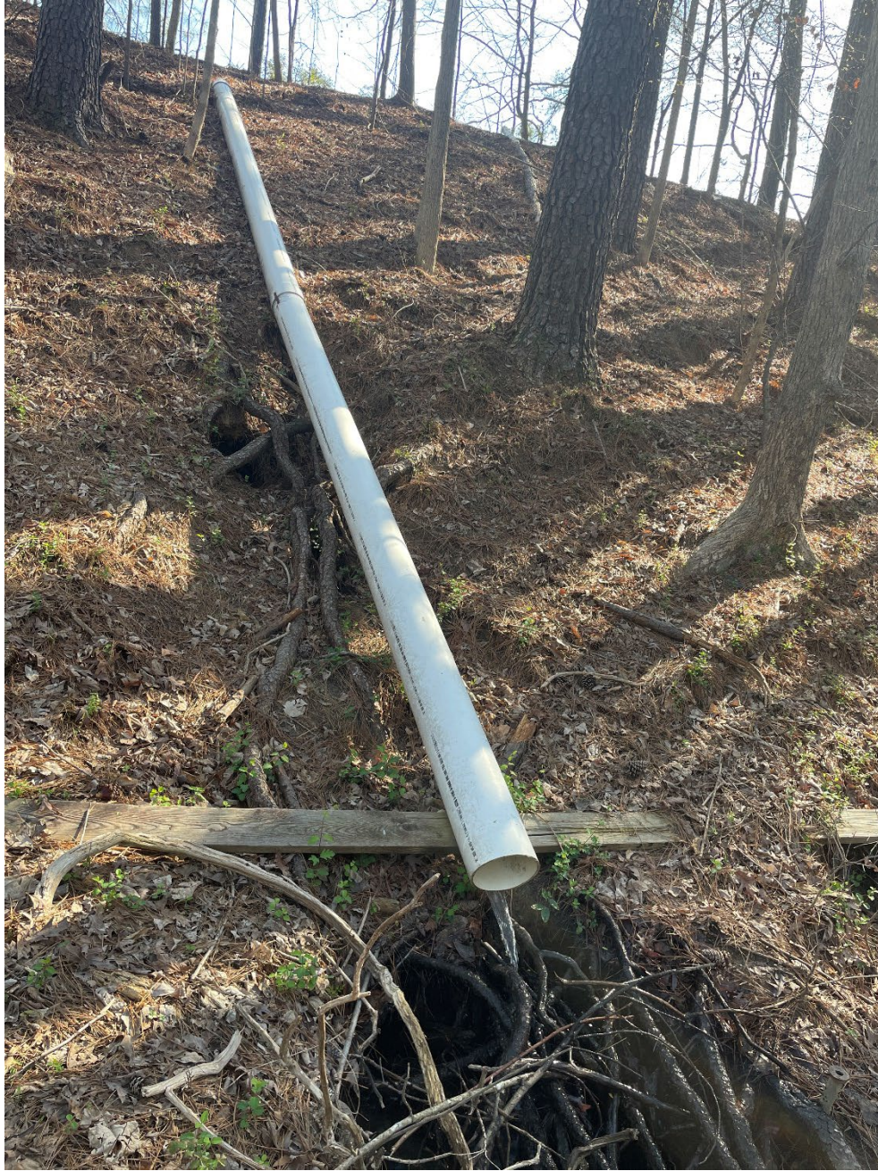
Photograph 6 – Overflow Device Outlet, Erosion Cavity Below Repaired Joint, Erosion Cavity at Outlet
