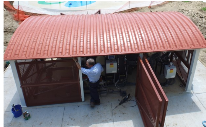
Recirculation mechanicals need to be protected in a small shelter
