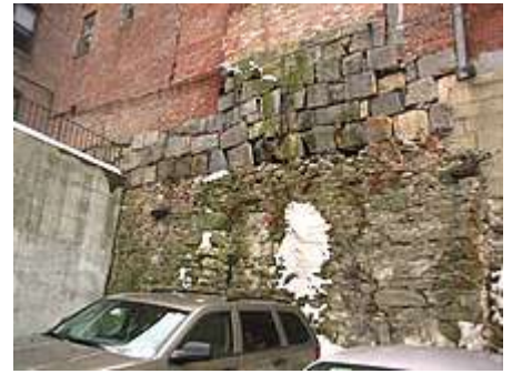
This wall in Beacon Hill, Boston , shows different types of brickwork and stone foundations
