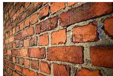
An old brick wall in English bond laid with alternating courses of headers and stretchers
