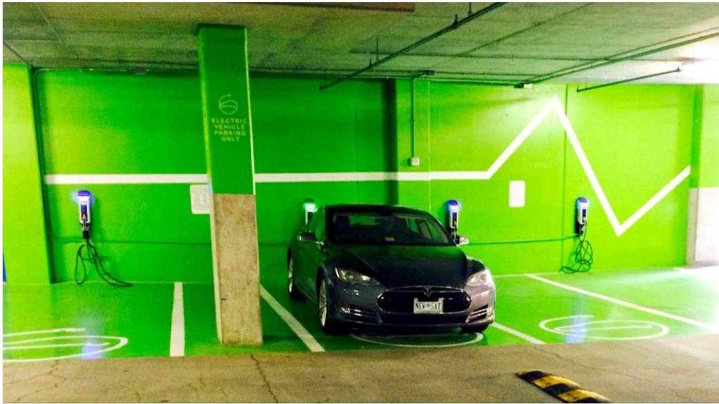
EV charging stations
