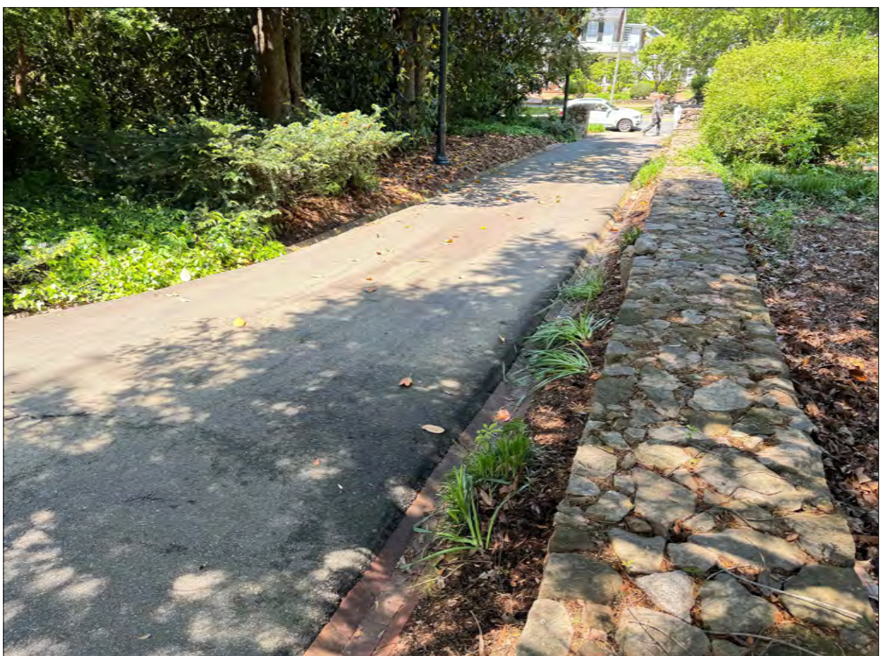
5. View of Driveway looking north showing existing stone wall on eastern perimeter (adjacent to Love House)
