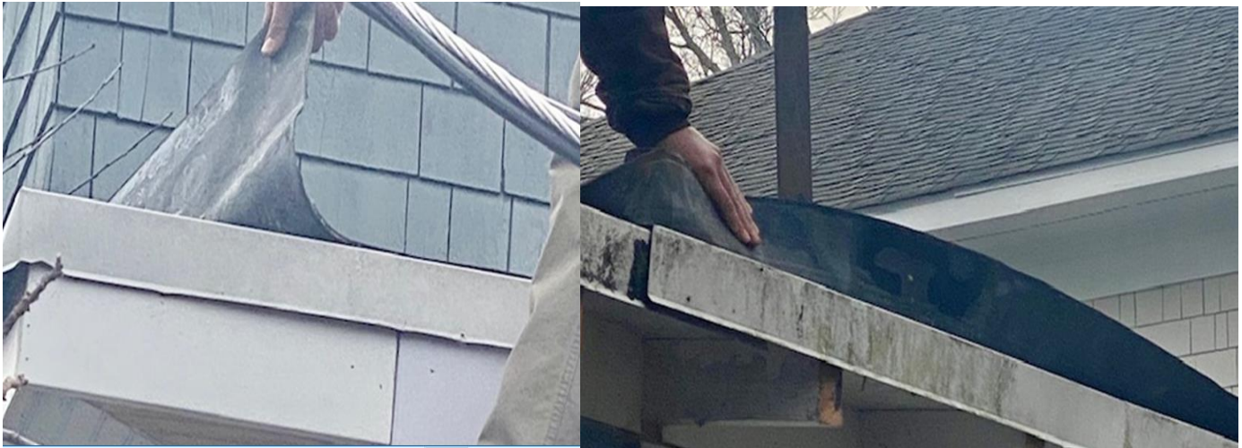
Views of Existing EPDM roof-current materials are not sealed around the perimeter nor on seams
