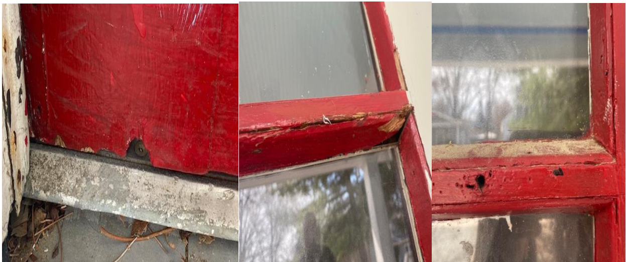
Poor conditions of existing front door
