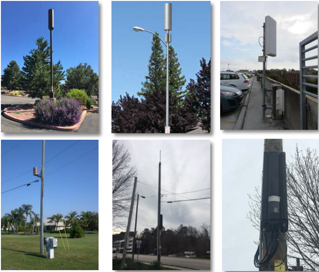
Figure 12: Small Cell Facilities - Single Node
