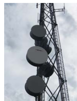
Figure 5: Microwave Dish Antennas
