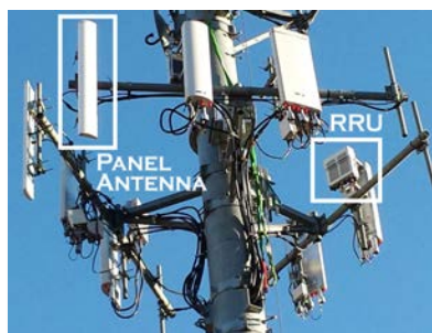
Figure 4: Panel Antennas with RRU's
