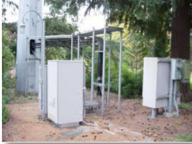
Figure 9: High Band Facility
