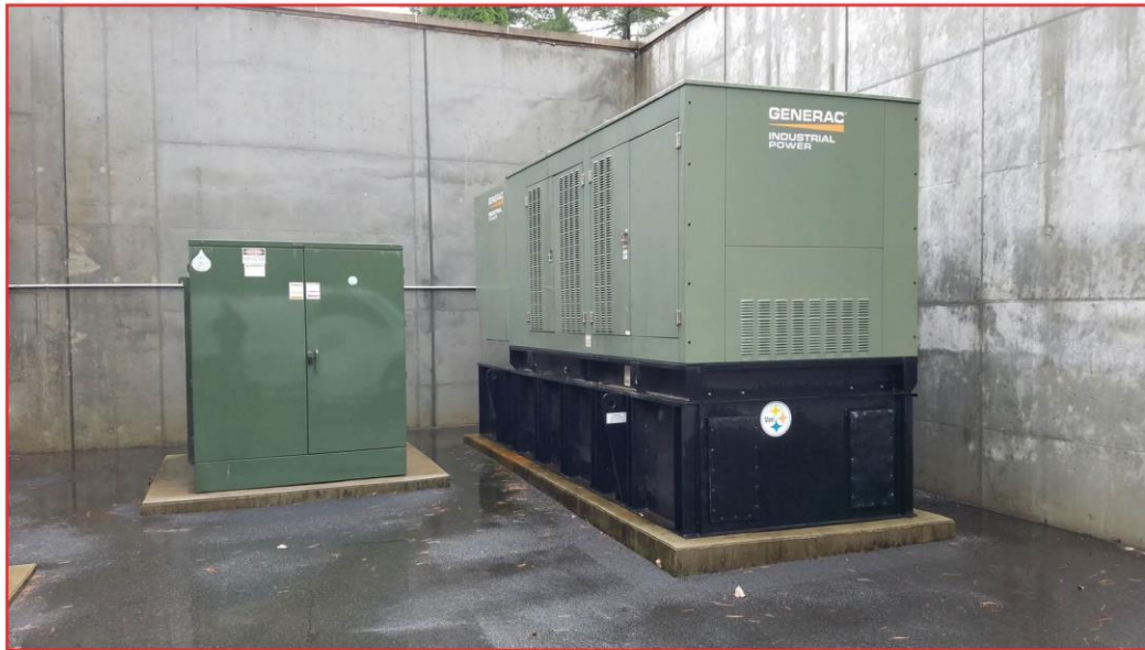
GENERATOR WITH ATTENUATOR AND SITE WALLS
