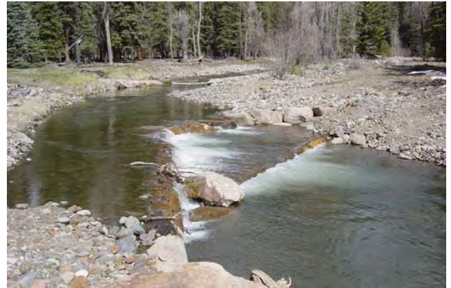
Figure 11-39 J-hook/log vane/log step with cut-off sill, East Fork Piedra River, CO
