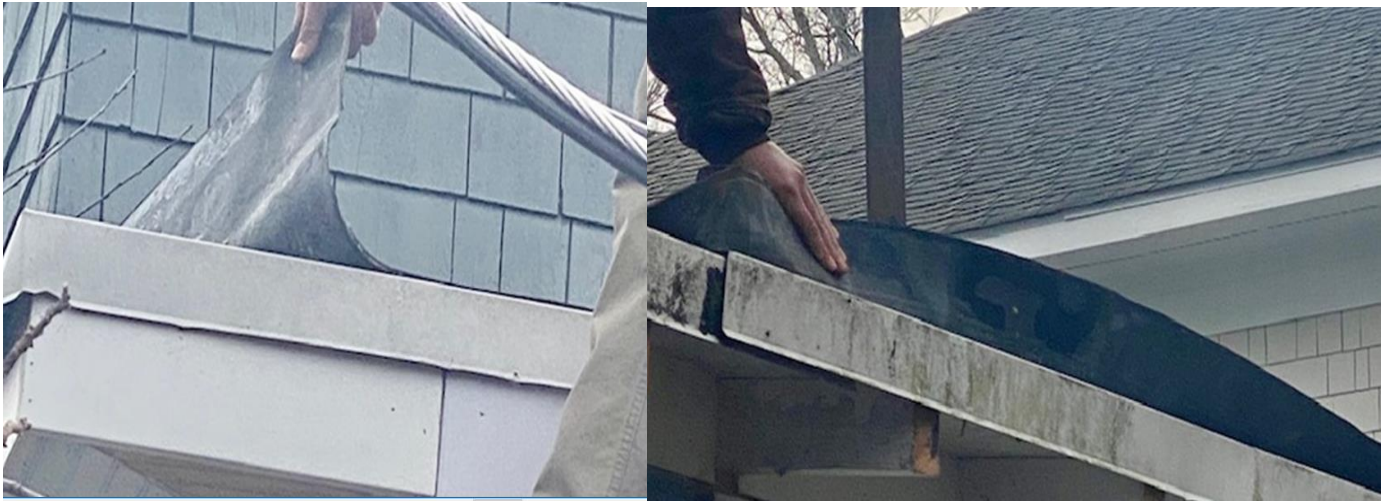
Views of Existing EPDM roof-current materials are not sealed around the perimeter nor on seams
