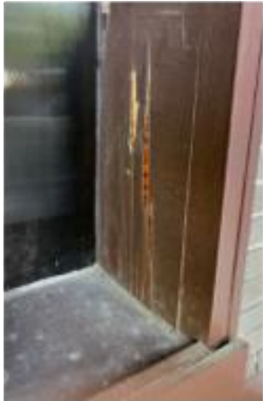
Example of delaminating surfaces
