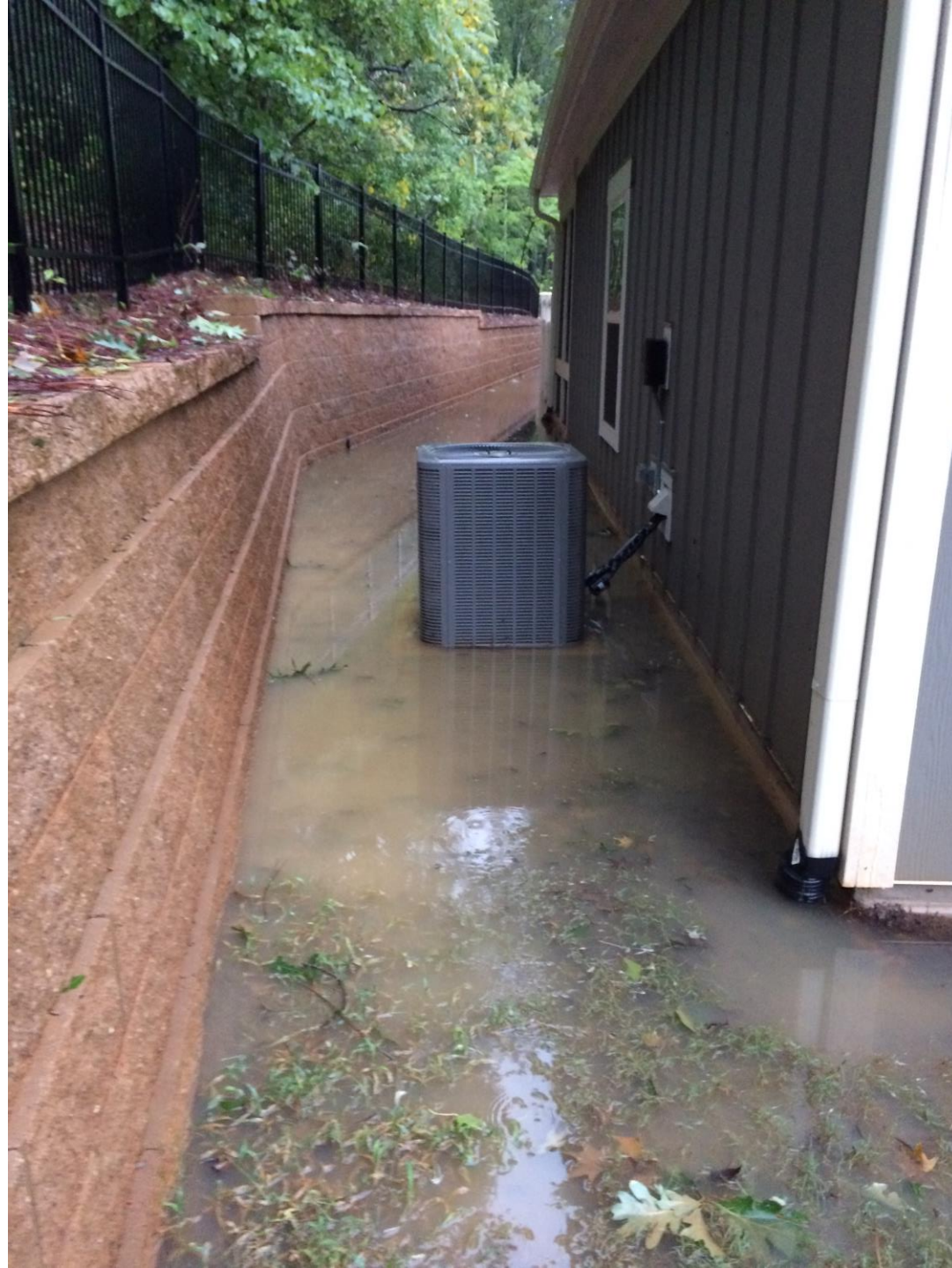
Flooding behind Lot 10 – Wood property to the left side behind the wall
