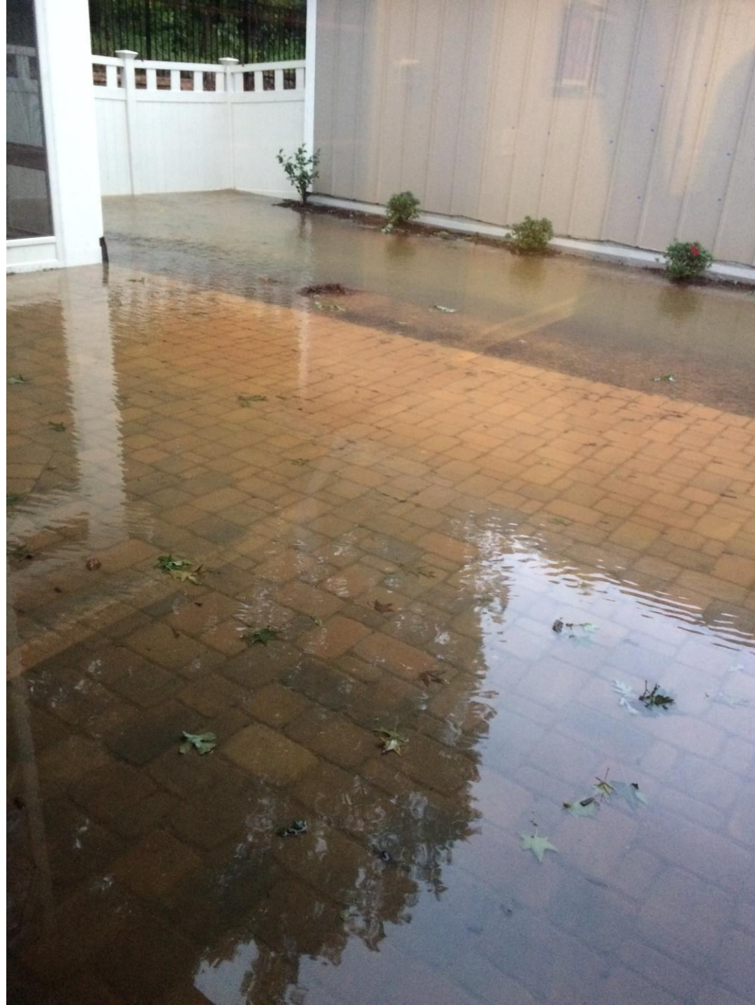
Flooding in courtyard of Lot 10 (also flooded inside this house)
