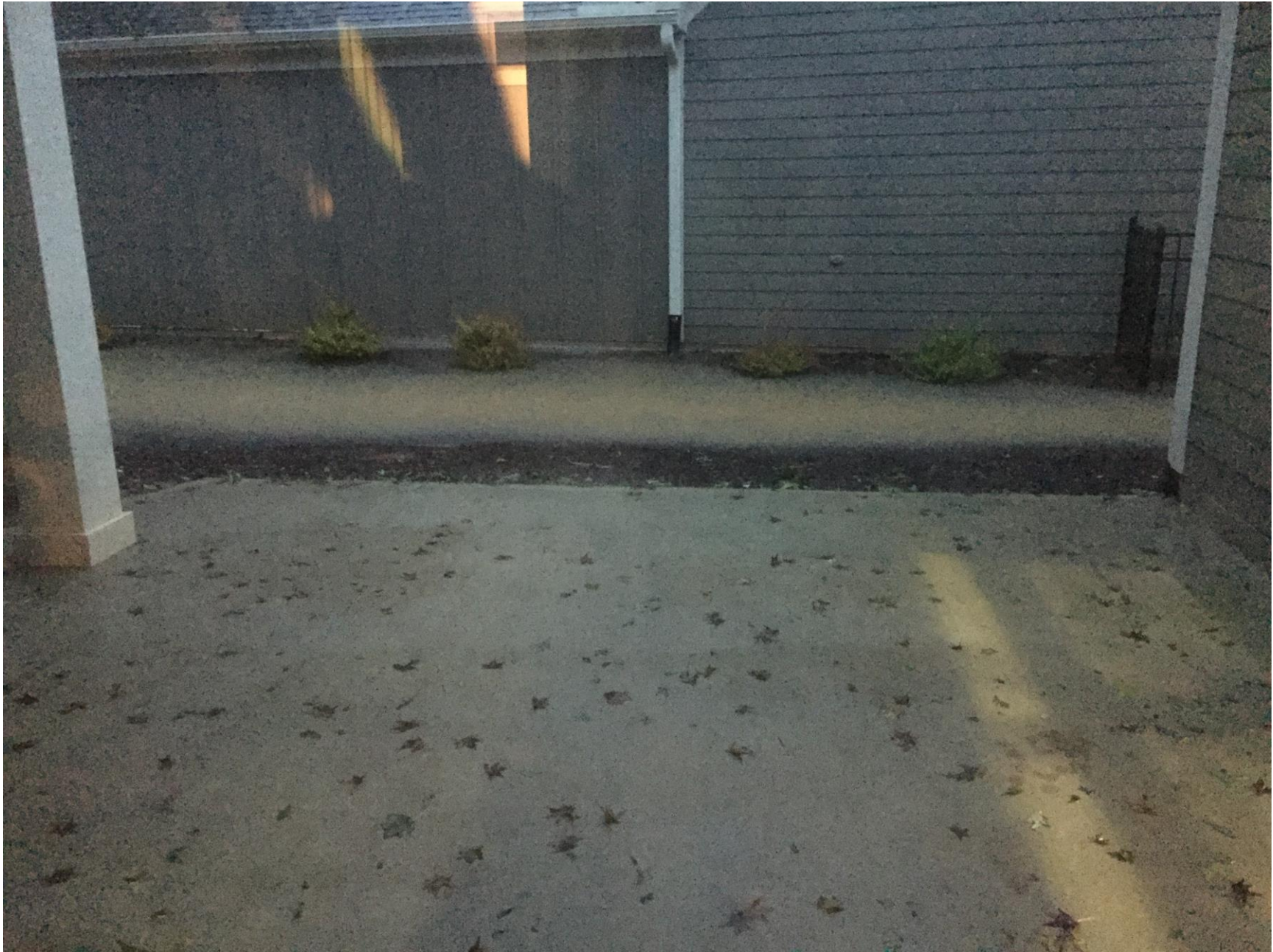
Flooding in courtyard of Lot 9
