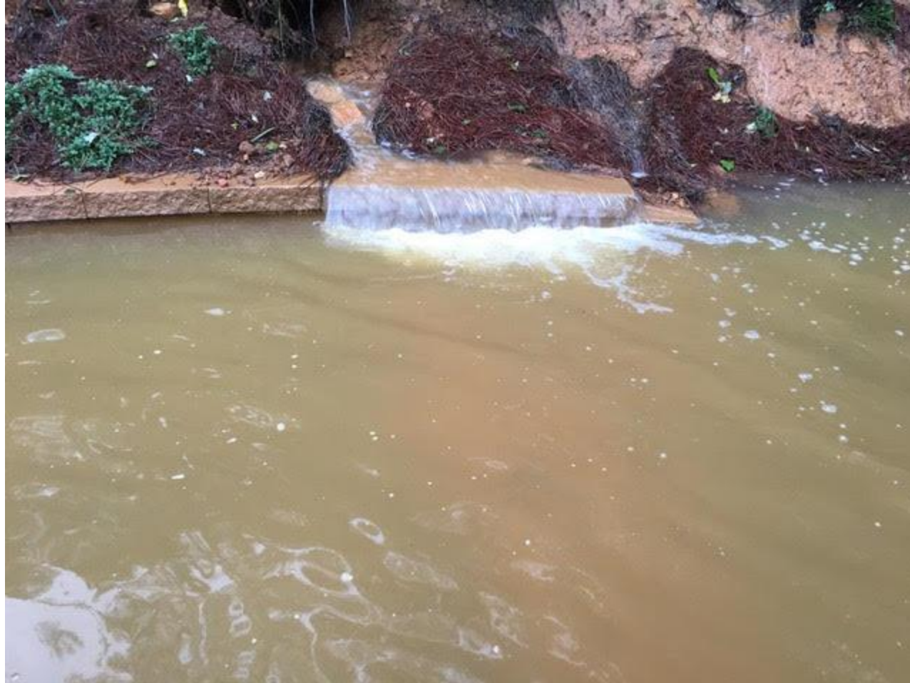
Run-off spilling over retaining wall coming from Wood property
