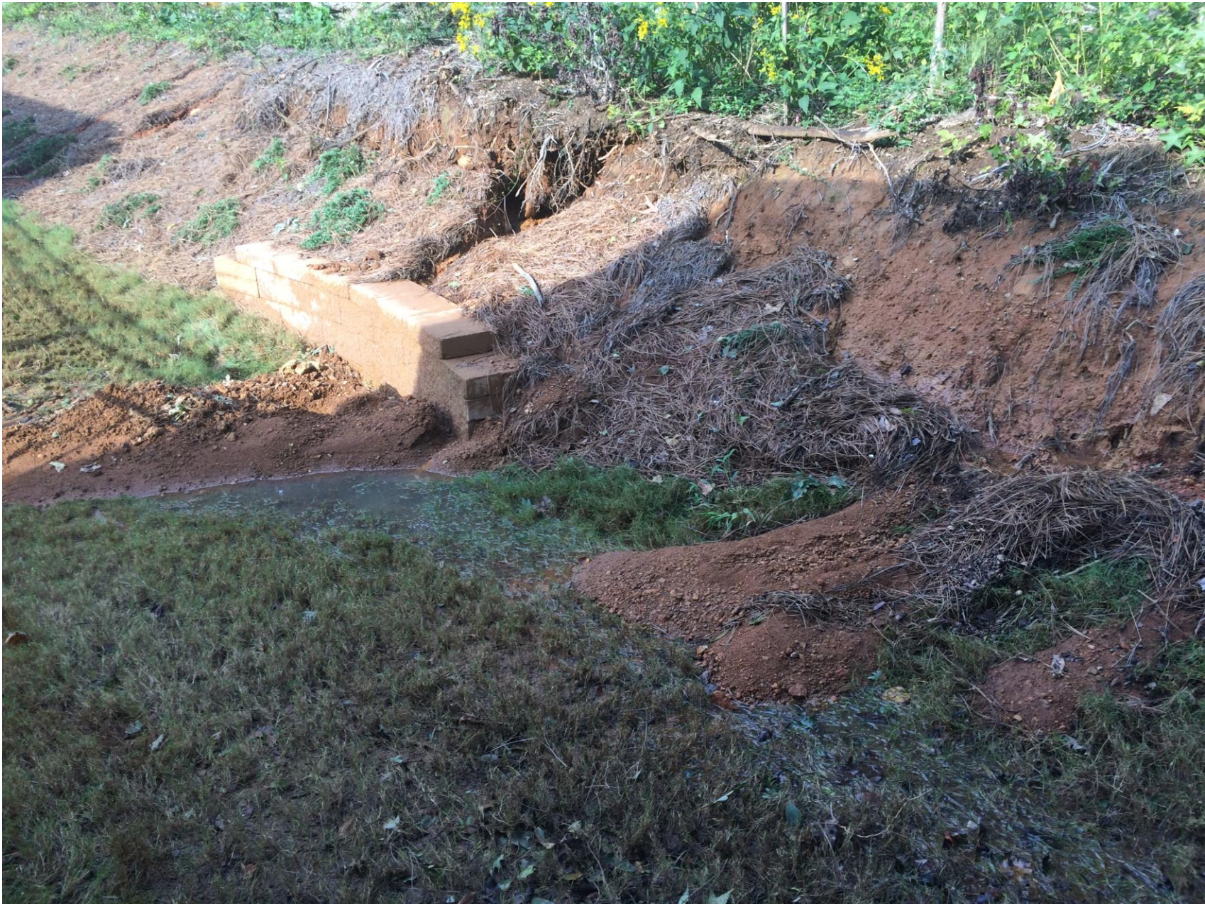
Accumulated mud/clay runoff from erosion of the slope behind lots 11 – 15 coming from Wood property
