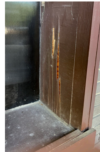
Example of delaminating surfaces
